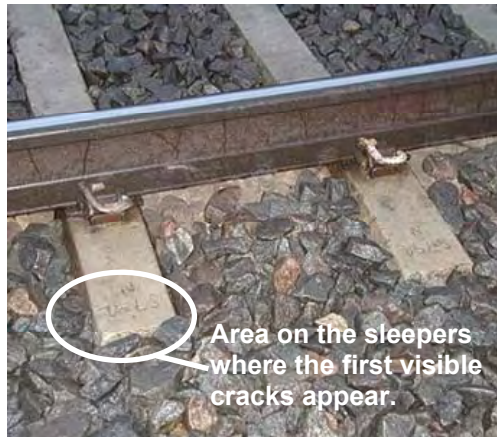
Figure 1 Picture showing how much of a sleeper that is visible when it is placed in the railway track and where the first visible cracks appear.
